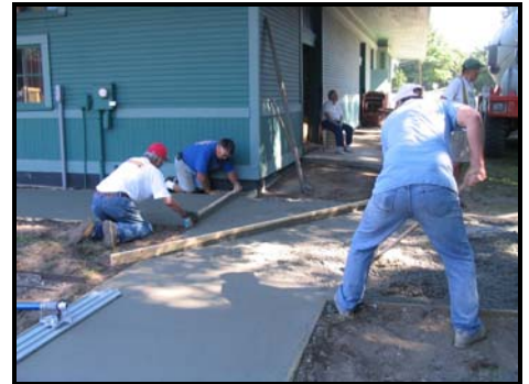
AV's Bill Weltyk, Hod Hunt, Bill Miller and Paul Delange smooth concrete at the Depot. Check it out!
