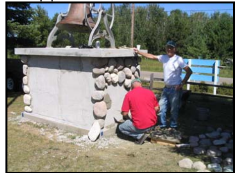
AV members Rick Teague and Dale Henry place stone on the Bell Tower at the Community Center
